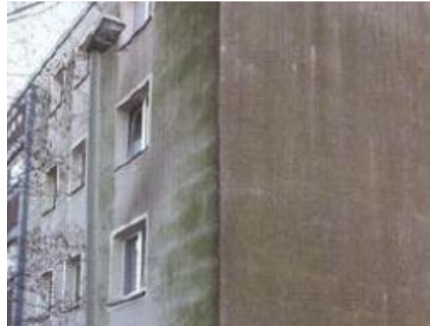
Figure (12) shows the facade of the building, which shows the accumulation of bacteria. 14
